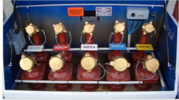
Cross-over-prevention and overfill prevention on a petrol-station filling point | © Secu-Tech
